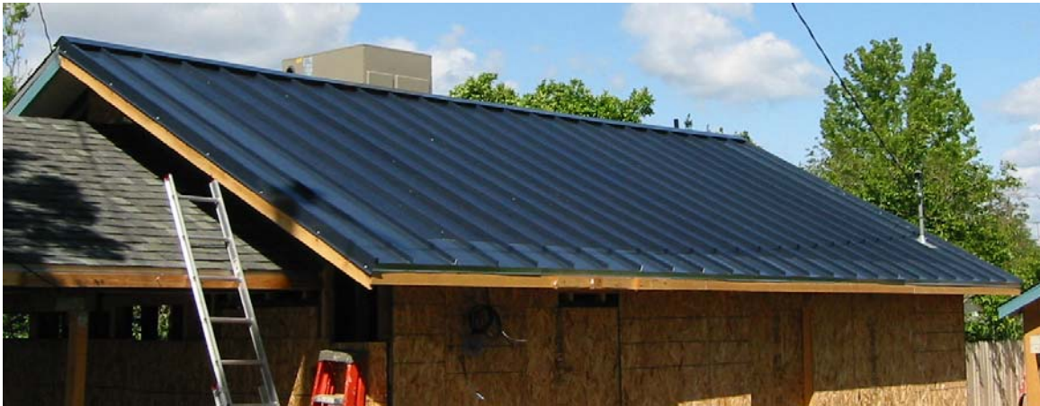
Habitat for Humanity/Uni-Solar project in Sacramento CA
