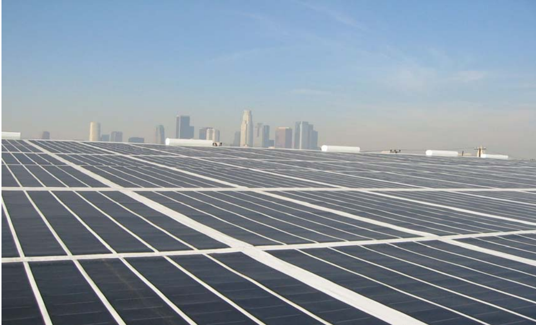
Solar Integrated Technologies (SIT) project in Los Angeles CA
