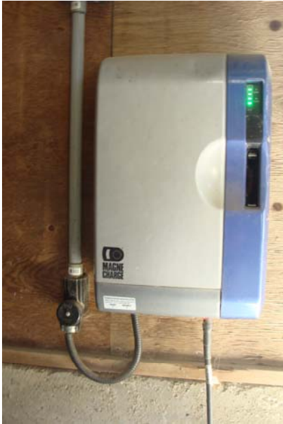
Wall mount charger plugged into a 14-50R, 240V receptacle.
